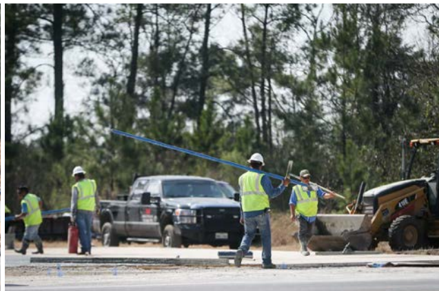
Construction continues on the TexCom site on Monday, Feb. 13, 2017, off of FM 3083 and Jefferson Chemical Road
