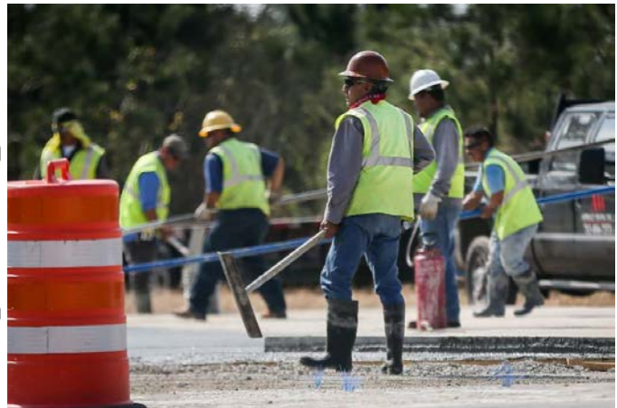
Construction continues on the TexCom site on Monday, Feb. 13, 2017, off of FM 3083 and Jefferson Chemical Road.
